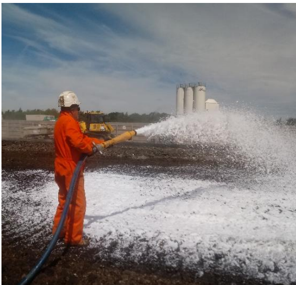
Photo 8.1 – Foaming soil with a neutral odour suppressant can reduce odour potential
