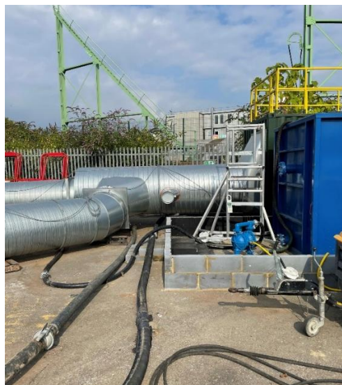
Extraction to odour control unit
